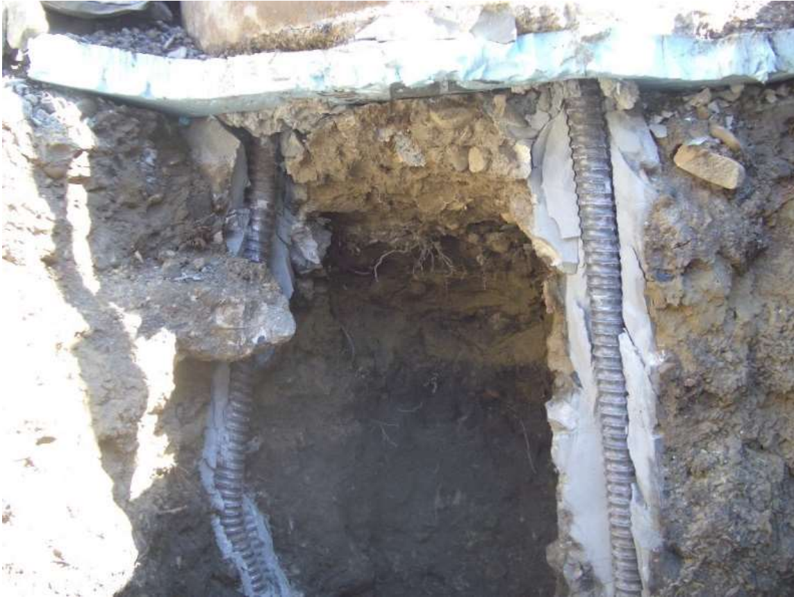
Figure 11: Hollow Bar Micropile Failure in Bending
